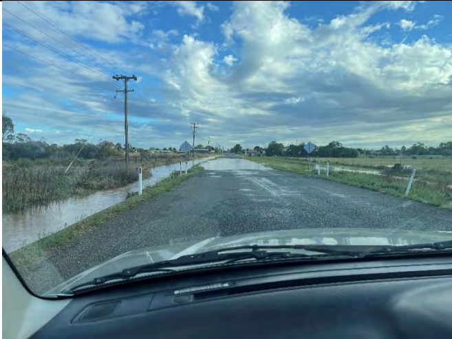
Plate C2.5 – (Time of photo unknown) – Looking north along Wargin Road from the Main Drain.
