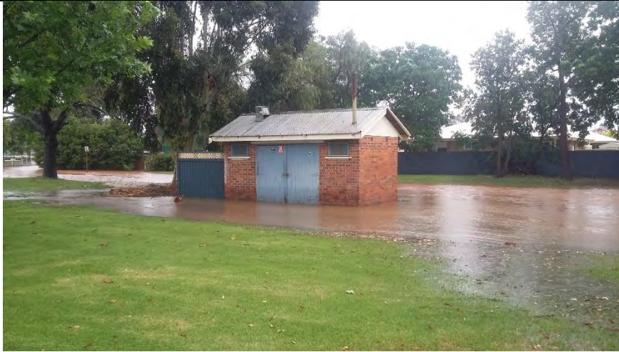
Plate C1.5 – (Photo taken at 10:00 hrs) – Floodwater surrounding building in Barnado Park.
