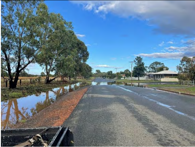
Plate C2.1 – (Time of photo unknown) – Floodwater inundating Cassin Street between its intersections with Compton Road and Mallee Street.
